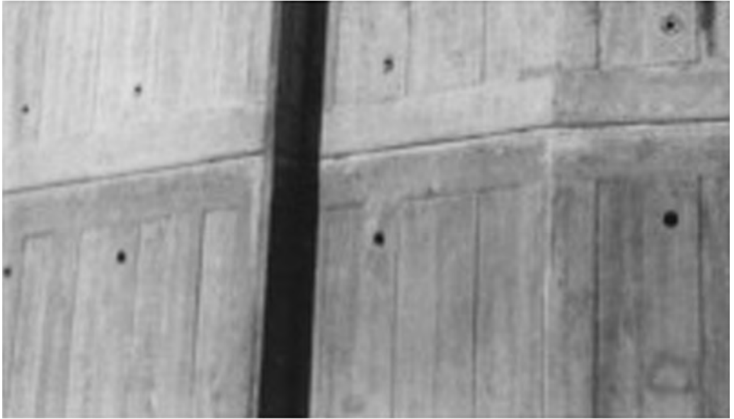
Concrete finish showing position of bolts. Source: Photograph courtesy of Rod Bond
